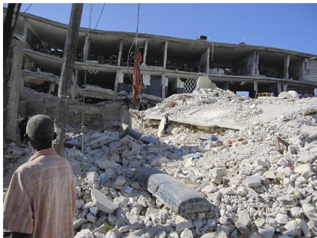
Figure 1. An onlooker views what is left of a large collapsed building in Port-au-Prince after the earthquake. The interior rooms are readily visible. Photograph courtesy of Colleen O'Connell.
